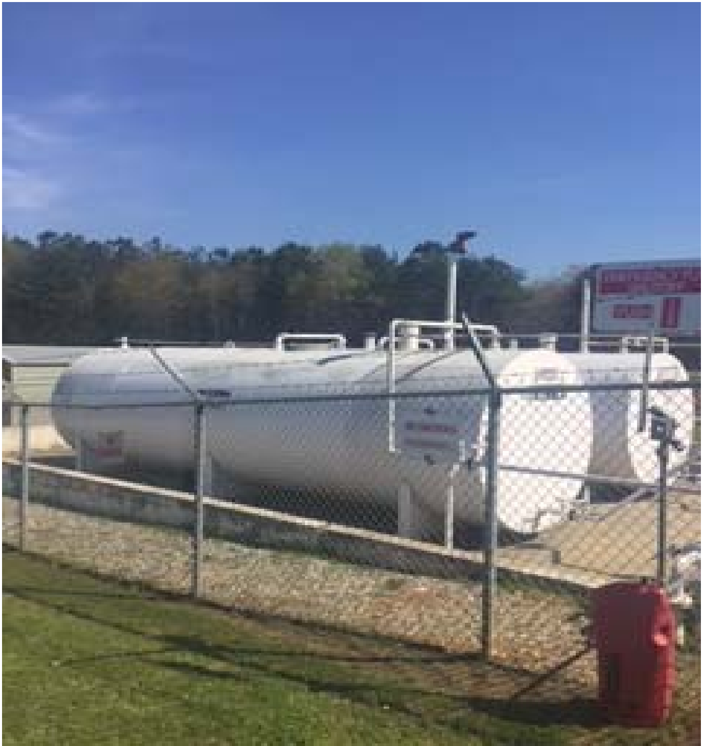
Fuel Farm and Containment Wall
