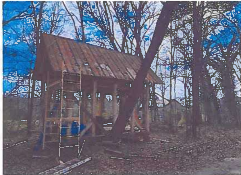
In January of 2025, we finished installing the roof of the restroom building.
