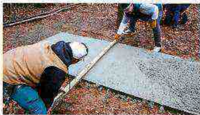
As you screed, you may need to fill in low areas with excess concrete.
