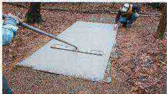
Flatten the concrete to force rocks down. It will help with texturing.
