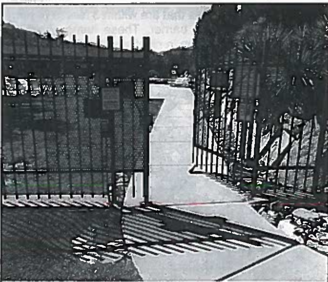
Commentary Figure 305.3 VIOLATION—WRONG SWING DIRECTION ON PEDESTRIAN ACCESS GATE
