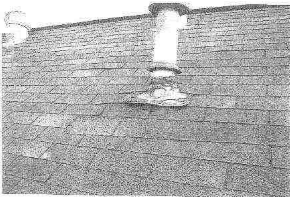
PHOTO 3B: View of joint flashing details and unfilled shingles adjacent to a metal vent.
