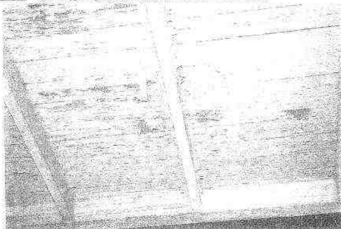
PHOTO 5B: View of typical paint delamination on exposed wood surfaces.
