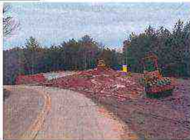
Cheohee Valley Substation Site
